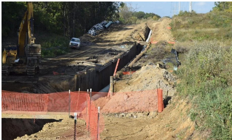
Image shows vehicles parking outside of the RoW boundary.
