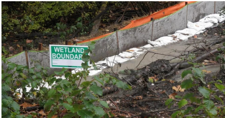
Figure 4: Wetland sign missing the name of the waterbody.
